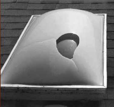
Old acrylic domes can be easily damaged.
