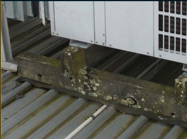
The Wrong Way
